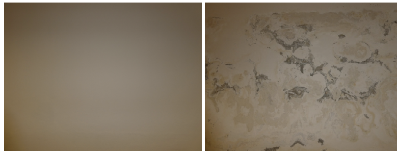
Fig. 1. Photos of the dry (left) and wet (right) parts of the wall
